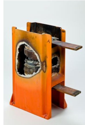
Failed Vacuum Interrupter Figure 4
